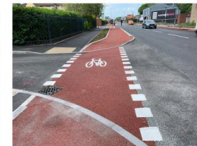
Priority to cyclists can be provided at side roads even in industrial areas using coloured surfaces and markings.
